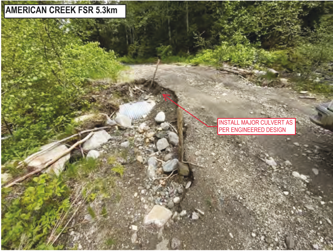
PHOTO 3 - FACING TOWN AT 5.3KM - PARTIALLY PLUGGED TWIN CULVERTS, ROAD EROSION AT OUTLET INSTALL NEW CULVERT AS PER ENGINEERED DESIGN
