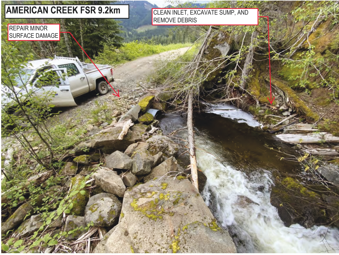
PHOTO 4 - FACING TOWN AT 9.2KM - CULVERT FUNCTIONING, PARTIALLY PLUGGED CLEAN INLET, EXCAVATE SUMP, REMOVE DEBRIS. REPAIR MINOR SURFACE DAMAGE ALONG ROAD
