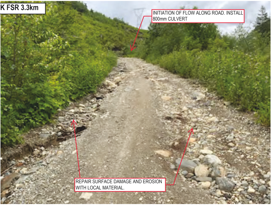
PHOTO 2 - FACING WOODS NEAR 3.3 KM - DAMAGED SECTION OF ROAD DOWN CHAIN FROM CULVERT RE-ESTABLISH ROAD PRISM AND REPAIR SURFACE DAMAGE WITH LOCAL MATERIAL.
