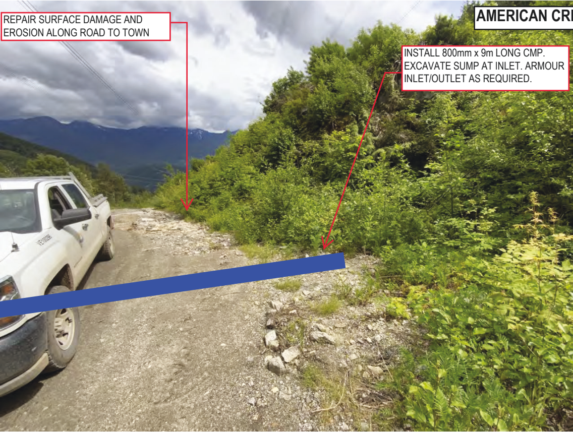
PHOTO 1 - FACING TOWN AT 3.3KM - PLUGGED CULVERT, INLET. WATER FLOWED ALONG ROAD TO TOWN INSTALL NEW 800mm DIA X 9m LONG CMP CULVERT. EXCAVATE SUMP AT INLET. ARMOUR INLET/OUTLET AS REQUIRED.
